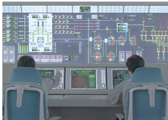
Central control room (for illustrative purposes)
